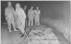
The 117-foot diameter tank required 20,000 square feet of fiberglass material. Two layers of fiberglass were laid to provide a new plastic type bottom.
